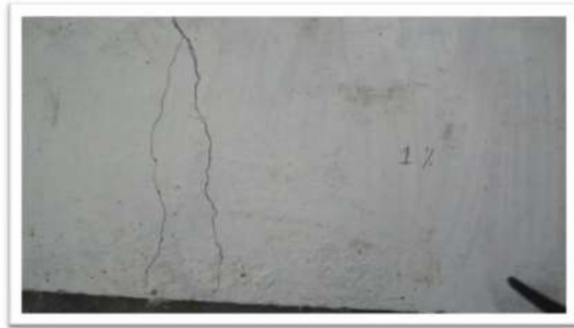
Fig 5.9 Crack Pattern in Ferrocement Panel
